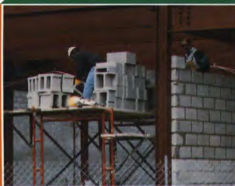
The construction workers begin to build one of the twenty-eight rooms of the new addition.
